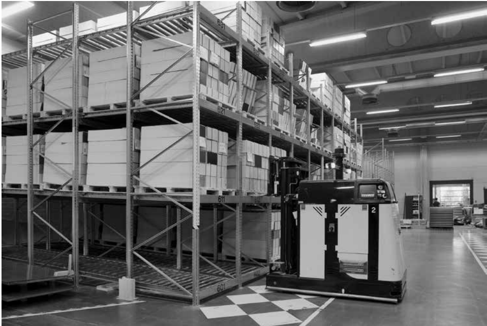
Figure 19.4 Robotic fork-lift truck serving push-back roller racking
