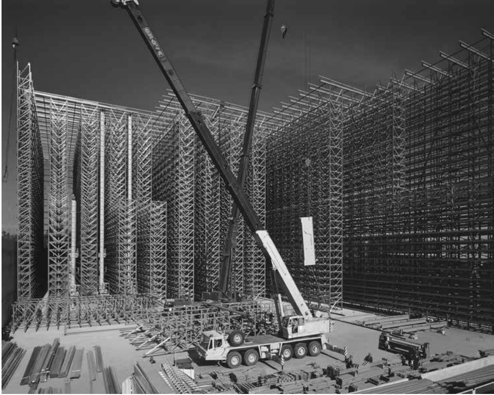
Figure 23.5 Rack-clad warehouse under construction showing pallet racks and AS/RS cranes within the racks
