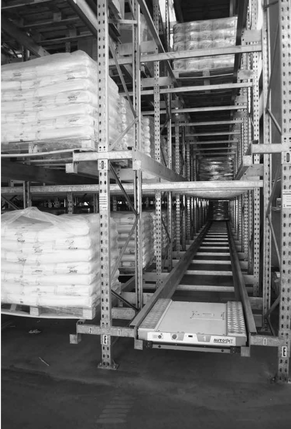
Figure 19.6 Shuttle racking, showing a pallet shuttle placed in the first rack position at low level
